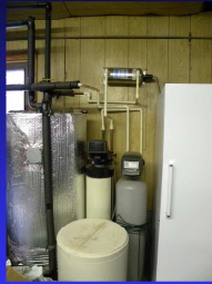
System in Garage – Two Rooms Away from the Pressure Tank
