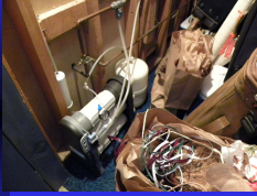
Reverse Osmosis Unit – Basement Closet on the Floor
